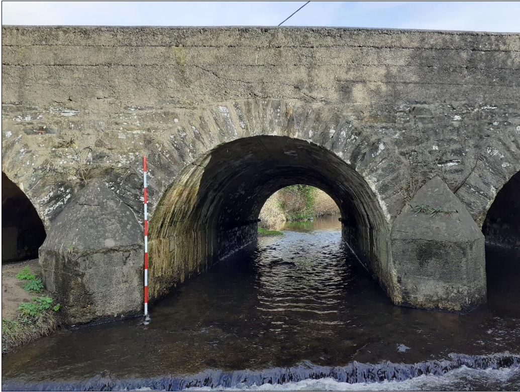
Plate 5: West (downstream) elevation of Burnfoot Bridge showing concrete plinth, cutwaters and parapet, and cut stone voussoirs, facing east
