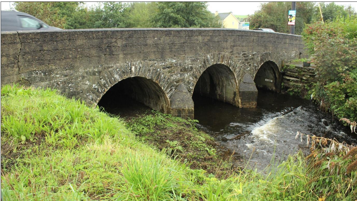
Plate 4: West elevation from north with stone arch and spandrel masonry over mid twentieth-century cast-concrete arch extensions. Parapet, cutwaters and paved river bed are also all of cast-concrete.
