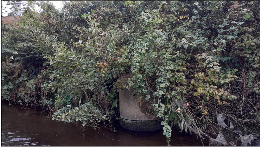
Plate 19: View of south bank of river and cylindrical concrete pipe approximately 30m west (downstream) of Burnfoot Bridge
