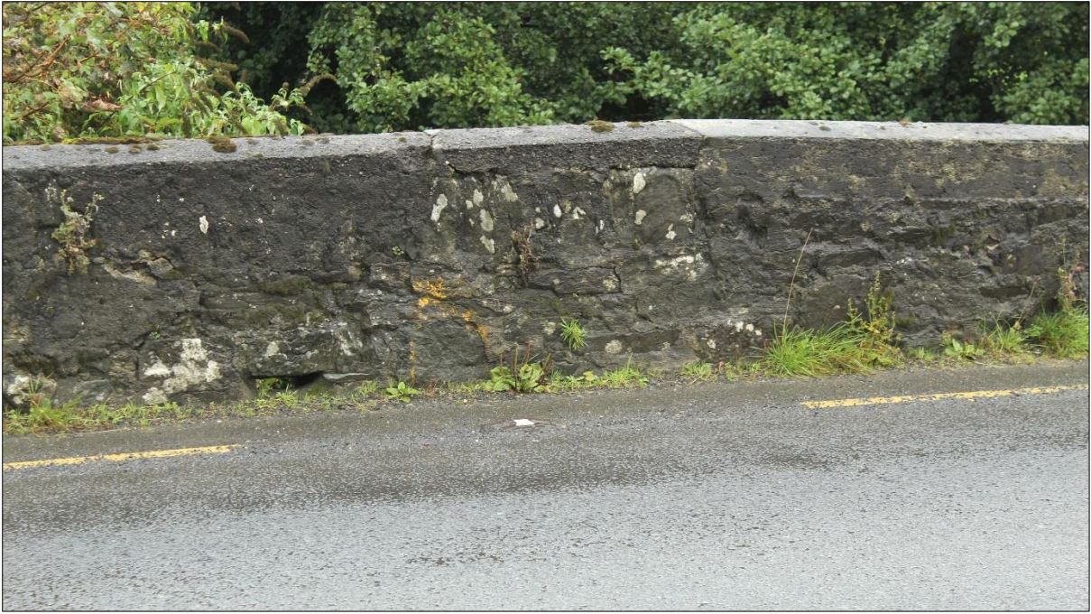
Plate 3: Road-side detail of original, eastern parapet masonry to crown of bridge. Note drainage hole from bridge deck to left of centre of photograph and original vertical coping stones beneath, or replaced by cast-concrete capping.
