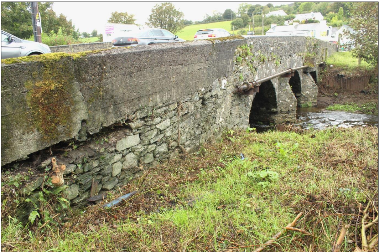
Plate 6: East elevation from south bank with cast-concrete extension to parapet masonry added when road approaches to bridge were raised during mid twentieth-century.
