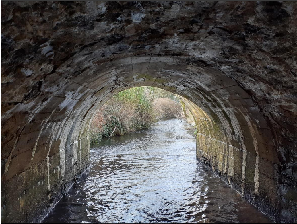
Plate 3: Bridge soffit, showing the composite construction of the widened bridge, facing west
