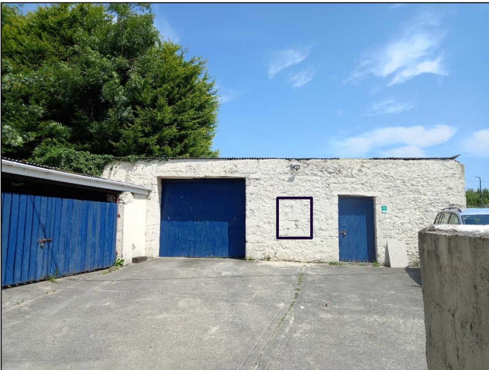
Plate 15.34: View towards east elevation of rear outbuilding within former RIC barracks complex. Note blocked up opening (black line) and breeze blocks with concrete lintels to existing opening surrounds. Note also attached modern built shed to northwest
