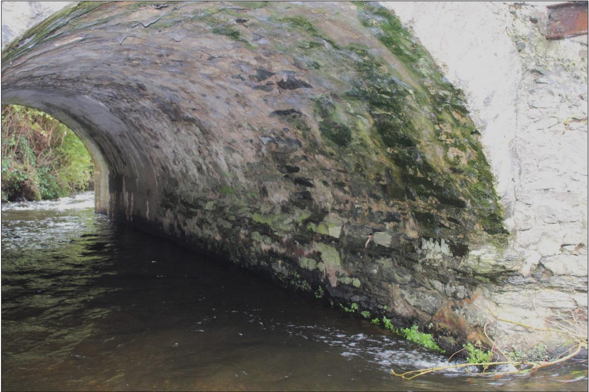
Plate 9: Detail of pier between southern two arches from east opening. Note extension of archway to west by approximately 50% in cast concrete.
